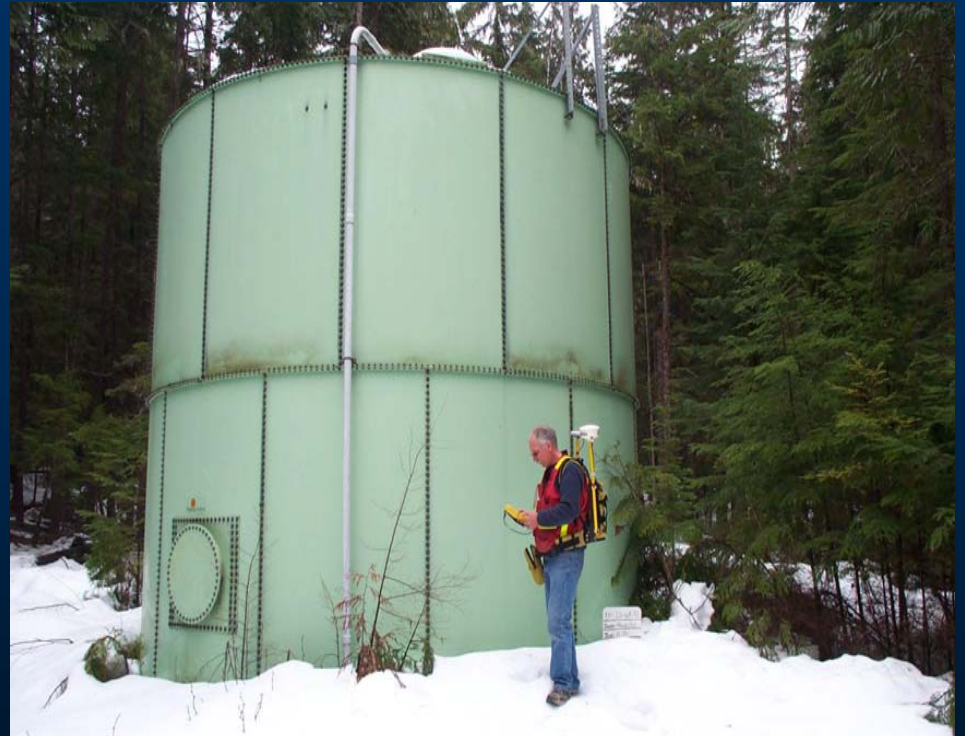
This is a storage reservoir at Mabel Lake Provincial Park (NO-LU-WAT-6-S-1)
