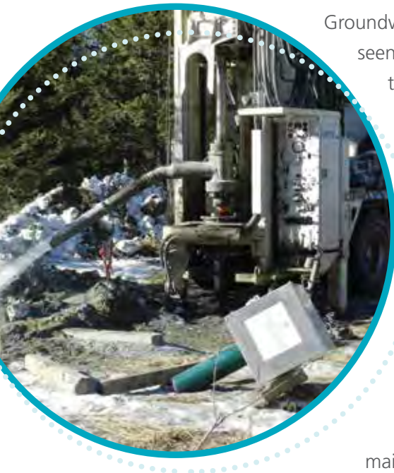
PHOTO: The OBWB, in partnership with several agencies, has successfully installed 12 groundwater monitoring wells to help track water supplies in Okanagan aquifers identified as sensitive.
