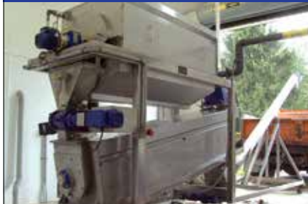
DSP Screw Press Model 3012, NY WWTP
